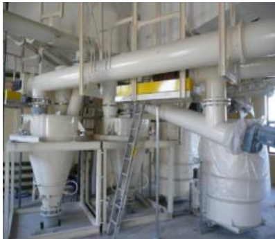
Automatic dosing of raw materials.
