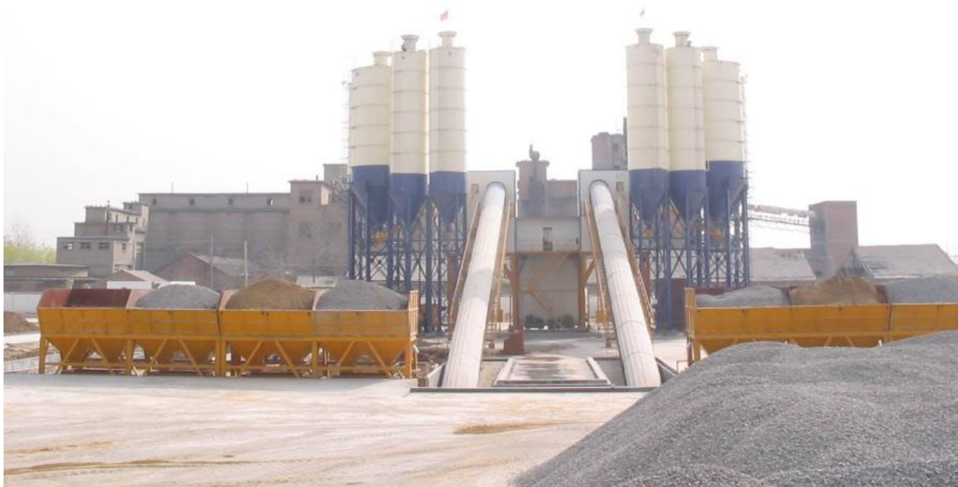
Double line of concrete mixing plant with 120 m 3 /h
